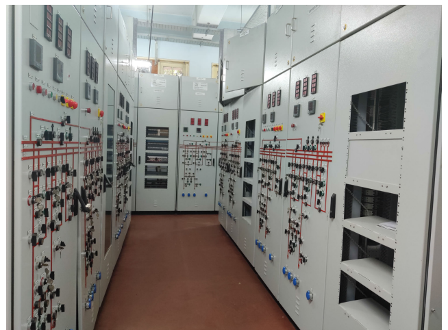
FIGURE 3. Six substations installed in the SESI-HTB.
