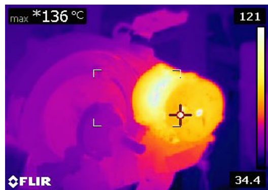
FIGURE 15. Infrared thermography of motor without filter configuration.
