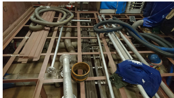
FIGURE 5. Pipes under metal floor.
