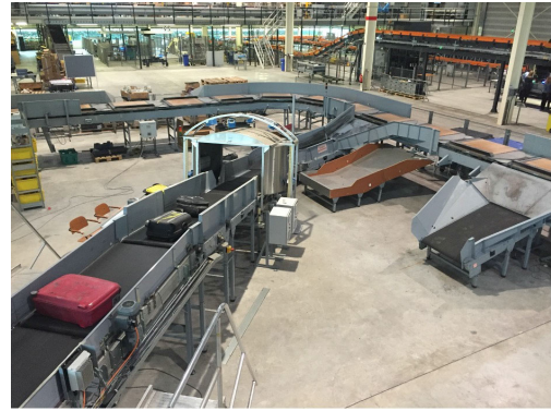
FIGURE 1. Belt conveyor system in an airport baggage handling transport system with multiple short conveyors.
