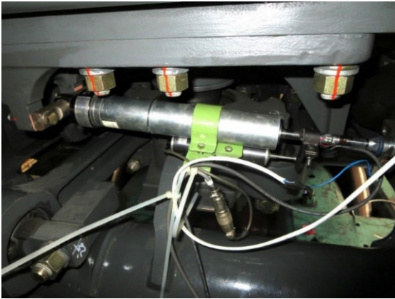
FIGURE 3. MR damper installed in the secondary suspension system.
