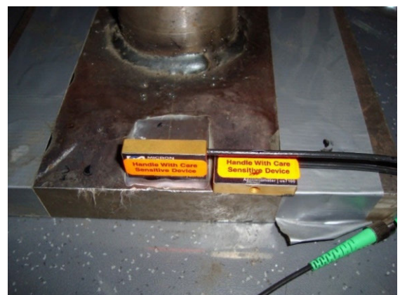
FIGURE 6. FBG accelerometers installed on the carriage floor in lateral and vertical directions.
