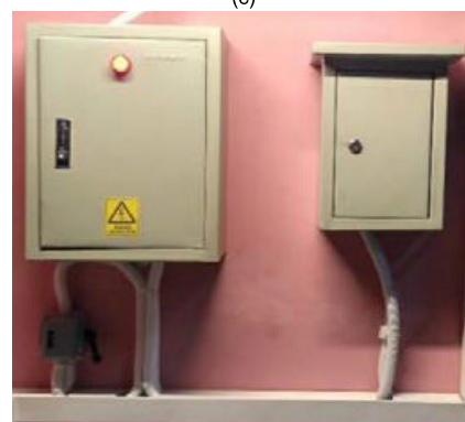
FIGURE 4. Main components of the implemented microgrid-interactive configuration; (a) solar modules, (b) battery units, (c) battery protection panel and hybrid inverter, (d) PV and AC protection panels.
