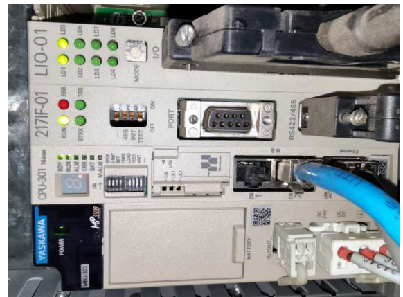
Hoisting motor drive system Trolley motor
