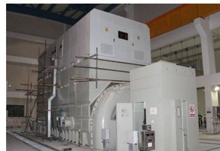
FIGURE 1. New 300Mvar SC.
