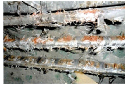
FIGURE 1. Stator windings aged for a long time due to internal discharge [5].
