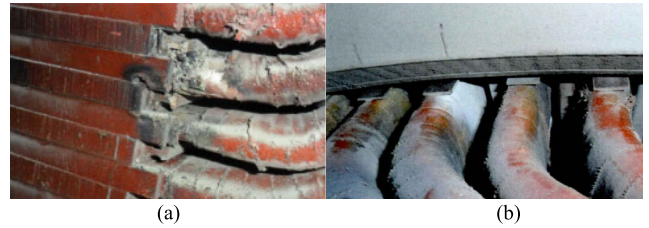
FIGURE 4. (a) Corona discharge at the slot outlet causes single phase ground fault on a 10kV three-phase asynchronous motor [18]; (b) Marks of corona discharge at the slot exit of a 2000kW/6kV high voltage motor [5].
