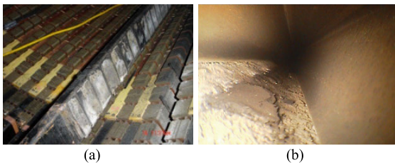
FIGURE 6. (a) The fault scene of the spark discharge after the stator bar near the neutral point of the winding is removed, (b) Borescope images of the side of a stator bar surface damaged by vibration sparking [23].
