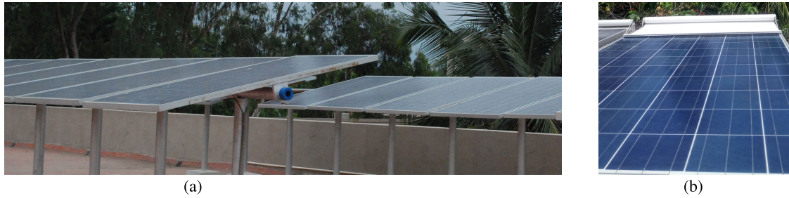
FIGURE 11. (a) PV array consisting of several 300 W polycrystalline PV modules. (b) Shading arrangement used for validating the GMPPT is shown as horizontal shading.
