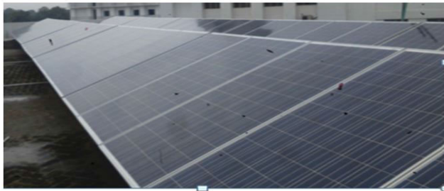
FIGURE 3. String of PV module of a 50 kW system.
