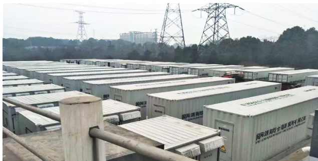
FIGURE 2. The Langli BESS project.
