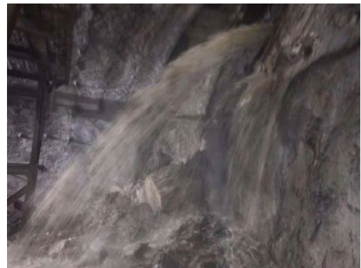
FIGURE 3. Water inrush from the upper left of the palm surface at YK21+122.8.
