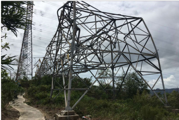
FIGURE 3. Collapsed tower in Guangdong due to the typhoon Tiange in 2017.
