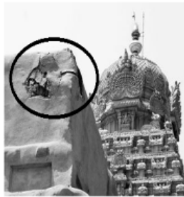
FIGURE 2. Brihadishvara Temple – Lightning strike chipped-off mortar in precincts adjacent to main tower (Sri Vimana) in 2011.
