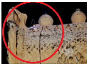
FIGURE 3. Brihadishvara Temple – Lightning strike damaged a sculpture in the top portion of the entrance tower (Keralanthagan gopuram) in 2018.
