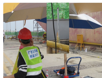
FIGURE 6. Bridge deck displacement test at lower end of suspender.
