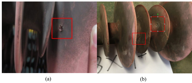
FIGURE 1. Shed holes of the composite insulators. (a) 550 kV composite insulator replaced from Tower #N242 of Line Xiaozong; (b) 220 kV composite insulator replaced from Tower #N25 of Line Huiqing.
