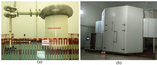
FIGURE 4. Test facilities at Electric Research Institute in Jiangsu, China. (a) AC power supply; (b) Fog chamber.
