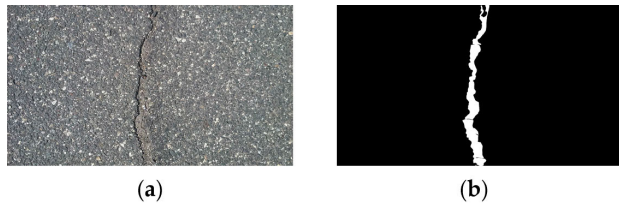
FIGURE 8. Crack500 data sample. (a) image; (b) ground truth.
