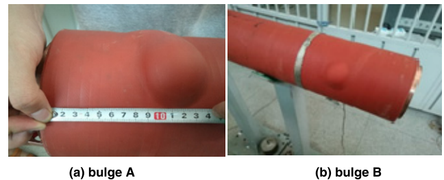
FIGURE 3. External bulge after sample insulation failure.
