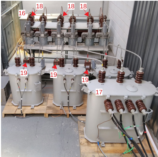
FIGURE 18. Test 13.8 kV substation.
