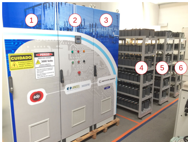
FIGURE 13. Photo of the developed equipment (1, 2 and 3) and the battery banks (4, 5 and 6).
