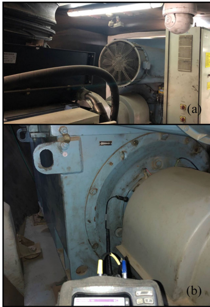
FIGURE 20. Vibration signal collection of the abnormal bearing.
