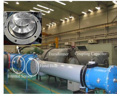
FIGURE 1. 220kV GIS test sample.
