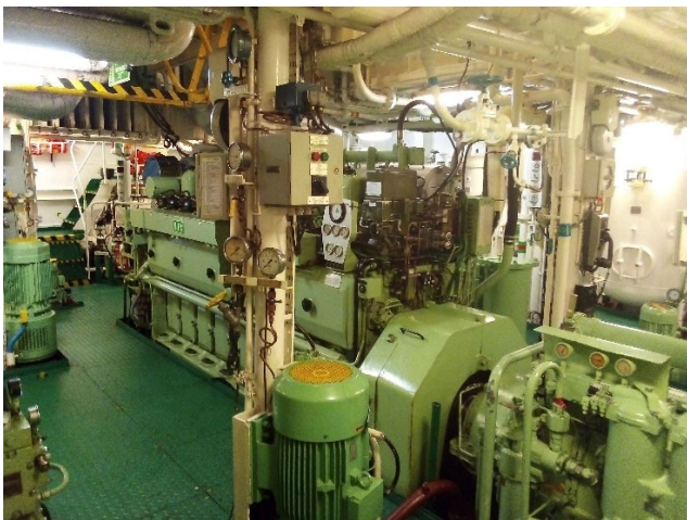
FIGURE 2. General view of the engine room on board Horyzont II.
