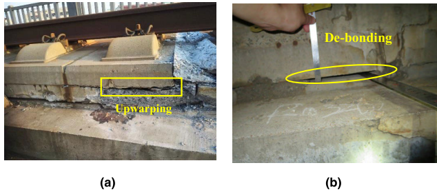
FIGURE 1. Typical defects of HSR slab track: (a) Upwarping; (b) De-bonding.
