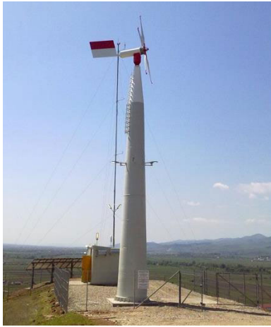
FIGURE 22. Wind turbine photo. SIHDC is installed inside the metallic container located behind the tower.
