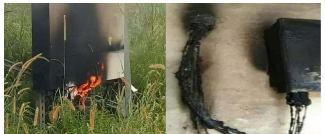
FIGURE 7. Damaged combiner box by fire [28].
