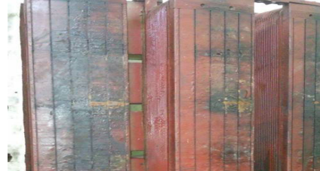
(b)Overheated ablated magnetic poles(a faulty generator in another hydropower station)
