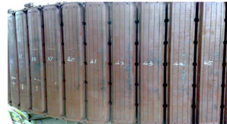
(a)Overheated ablated magnetic poles(a faulty generator)
