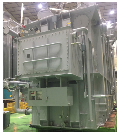
FIGURE 11. 105 MVA HV transformer for measuring load noise.
