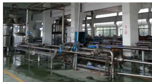
FIGURE 20. Photos of the flowmeter calibration site.
