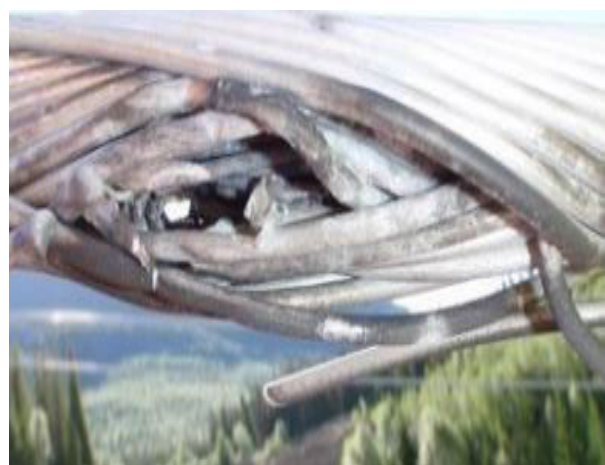
FIGURE 11. Lightning damage to conductor [105].
