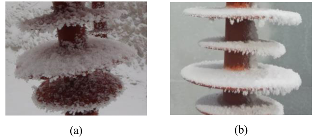
FIGURE 14. Observation of snow-covered insulators: (a) insulator in the field; (b) insulator in the chamber.
