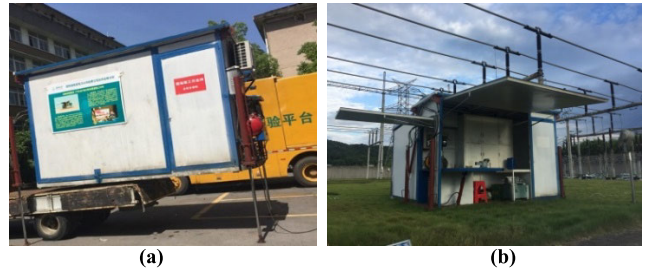
FIGURE 12. On-site application of the apparatus in the substation: (a) normality mode, (b) extension mode.
