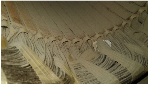
FIGURE 13. The view of a motor stator for PD measurement under contamination.
