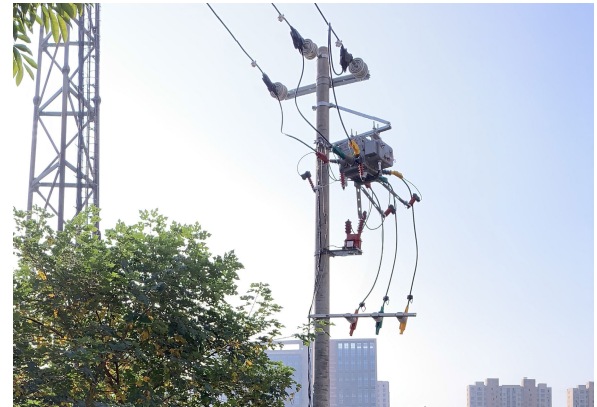
(a) Feeder terminal unit (FTU) added in the overhead line.
