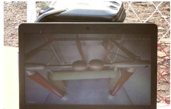
(c) The scene of arc grounding fault occurrence in the controlled arc discharge device.
