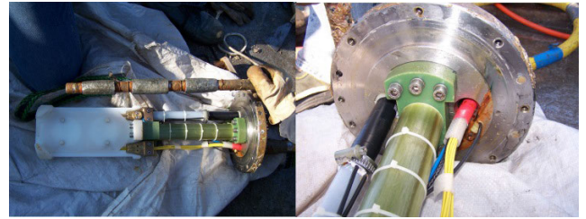
FIGURE 12. Pictures shows the interior of the Underwater termination box with rust showing the water level.
