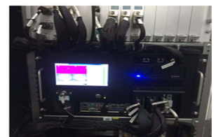
(b) Equipment in the control room
