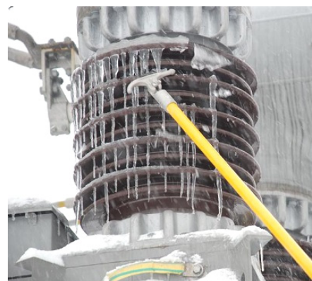
(a) Natural icing growth on substation post insulator
