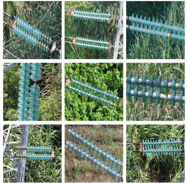
FIGURE 6. Images of insulators.
