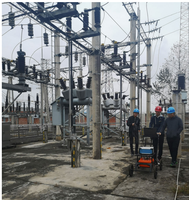
FIGURE 16. 110kv Transformer substation.
