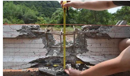
FIGURE 21. Mid-span vertical fracture of SJ-1.
