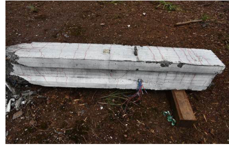
FIGURE 17. Right half span crack distribution of SJ-2.
