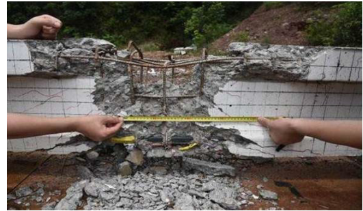
FIGURE 20. Mid-span transverse fracture of SJ-1.
