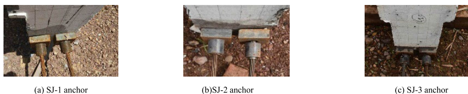
FIGURE 9. Anchorage falling off condition.
