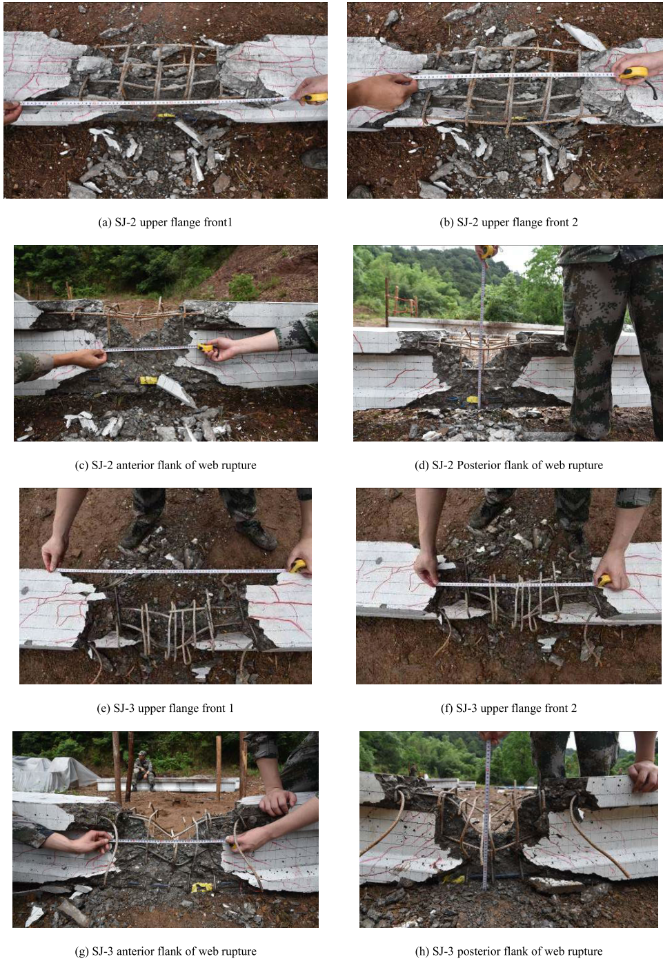
FIGURE 13. Photos of SJ-2, SJ-3 concrete breakage.
