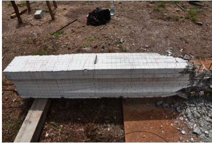
FIGURE 14. Left half span crack distribution of SJ-1.
