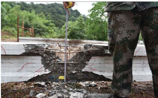
FIGURE 23. Mid-span vertical fracture of SJ-2.
