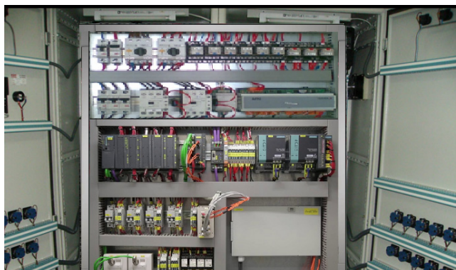
FIGURE 2. The power transformers measurement panel.
