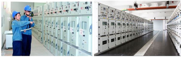
FIGURE 1. Line-of-sight human machine interaction in the power distribution room of the electrical substation.
