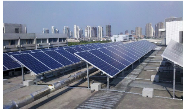
FIGURE 12. 10kWp distributed PV system for experiments.
