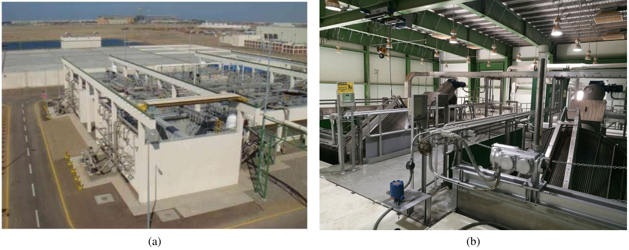
FIGURE 4. (a) Overview of the wastewater treatment plant; (b) Fine screen inside the headwork, where influent was filtered.
