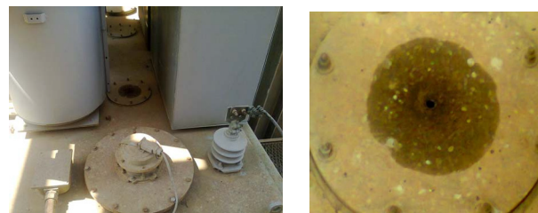
FIGURE 7. Atmospheric air leakage in the transformer under-study [43].
