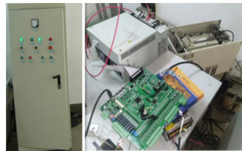
FIGURE 23. SW-PMLSM winding switching control cabinet and motor drive control module.
