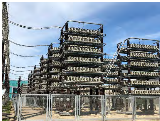
FIGURE 1. Filter capacitors in converter station.
