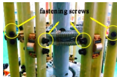
a. Normal working condition of moving contact
