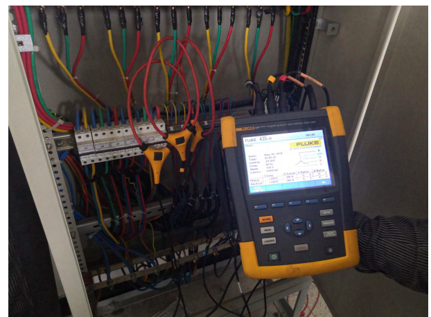
FIGURE 10. The field data acquired condition at campus substation.
