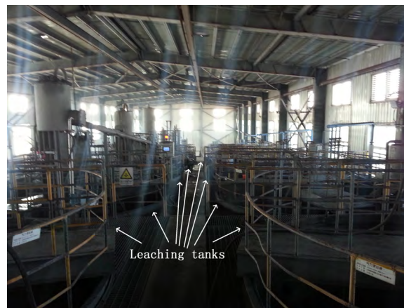
FIGURE 1. Photograph of the gold cyanidation leaching plant in a gold refinery.
